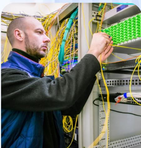
Telecommunication Network Deployment
