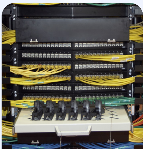
Structured Cabling System
