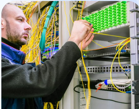
Telecommunication Network Deployment
