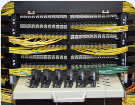
Structured Cabling System
